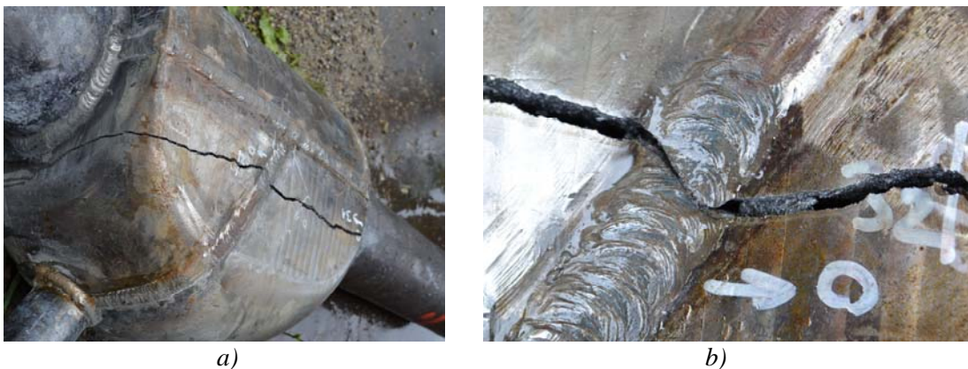
Figure 10. Position (a) and detail (b) of the crack after pressure test to destruction
